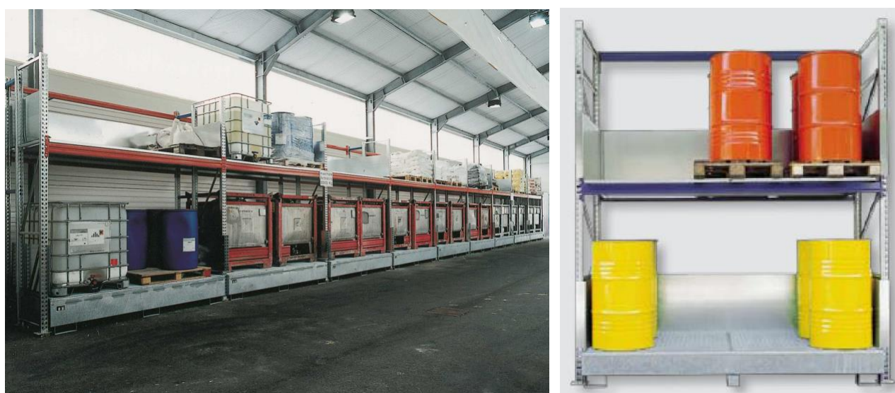
Figure 13: Examples of different types of shelving for hazardous waste containers
