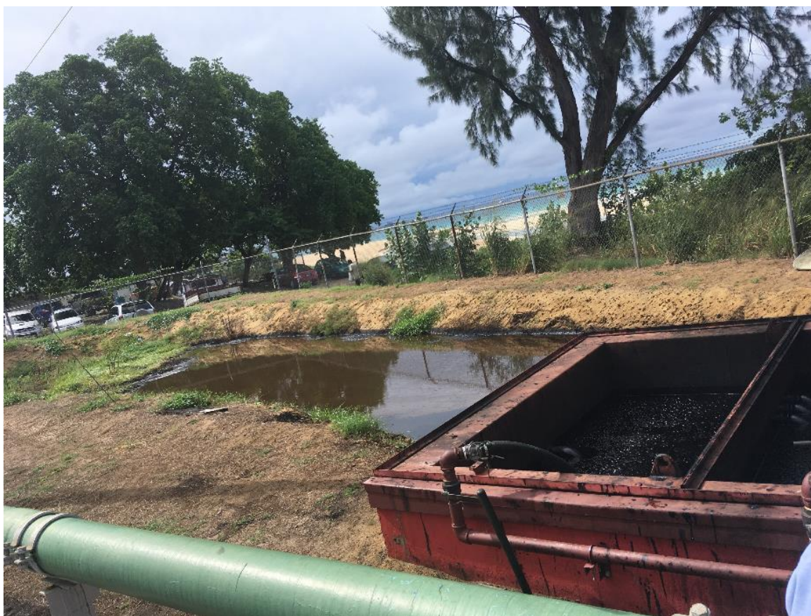
Figure 7 Non-functional oil-water separation tanks, prone to rainwater ingress and waste oil overflow in the environment (Photo: RWA Group, 2019)
