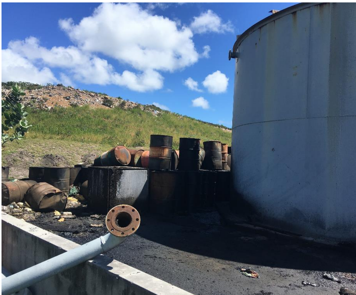
Figure 5 Waste oil storage in tank and drums, leaking in concrete containment bund (Photo: RWA Group, 2019)
