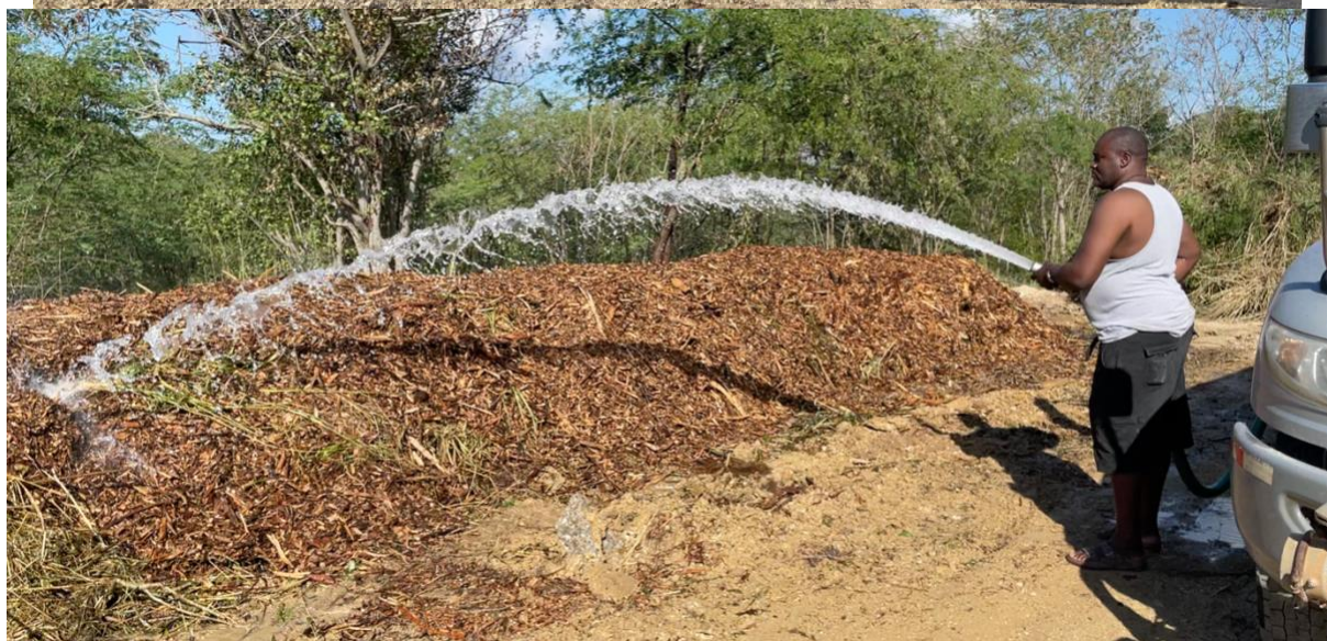
Continuously apply water as the layers are placed and the pile are built up.
