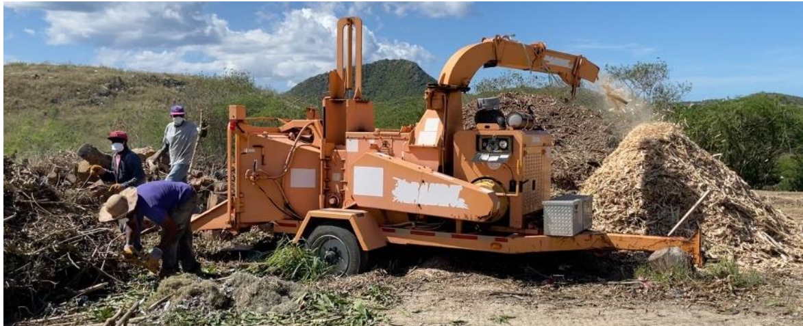
The larger material will then be processed through the on-site chipper. This is manually loaded and is therefore a slow operation, future investment is required into a machine loadable large shredder.
